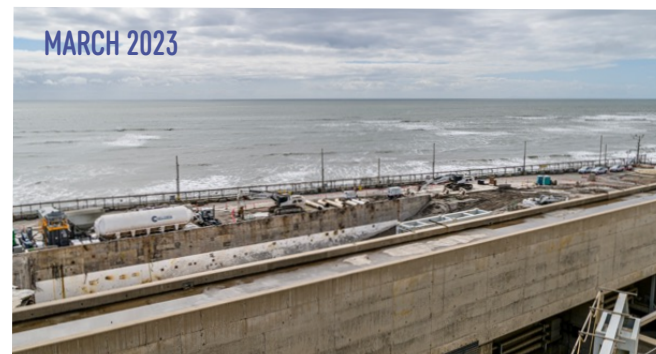
In two short years, the turbine structures and gantry cranes have been demolished
