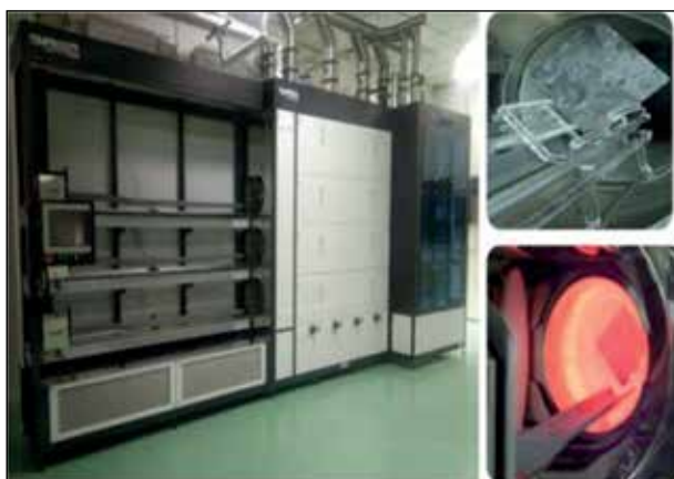
Fig. 7.11: Diffusion furnace installed at BHEL ASSCP (capable of processing POCl 3 & BBr 3 diffusion along with dry and wet oxidation)
