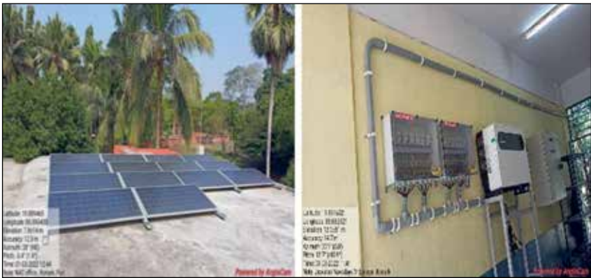
Fig. 3.6: Rooftop Solar Power Plant
