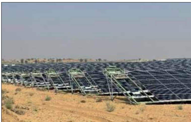
Fig. 10.21: 600 MW Solar projects installed under ISTS 1 tender
