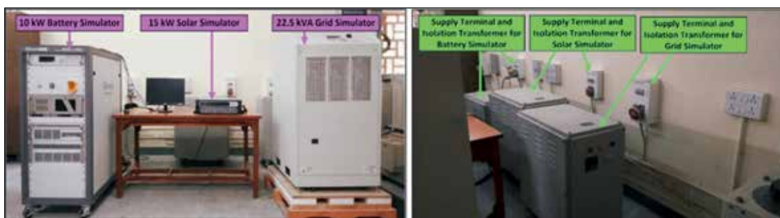
Fig. 7.6: A Comprehensive Test Bench comprising of Solar Emulator, Battery emulator, and an electronic load is developed to test solar inverters
