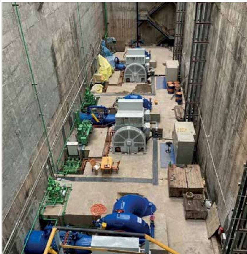
Fig. 4.5: Saptadhara Small Hydroelectric Power Project (3x6 MW) at Malkangiri, Odisha
