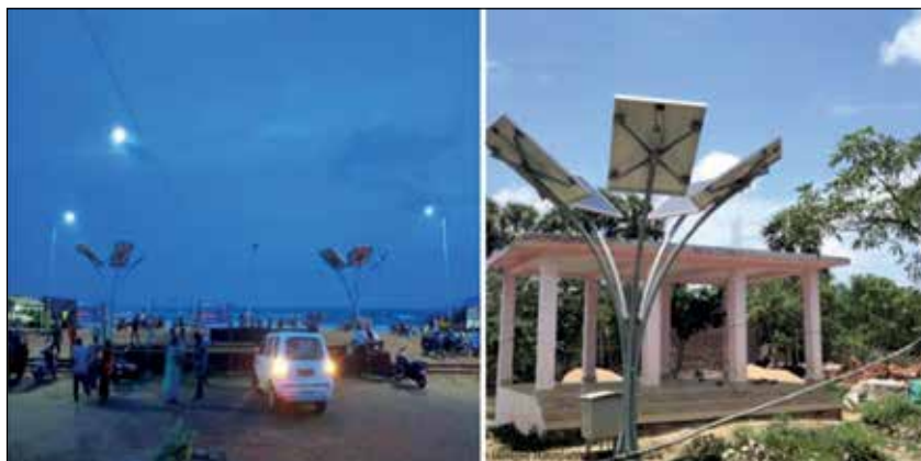
Fig. 3.5: Solar Tree and Street Lighting System
