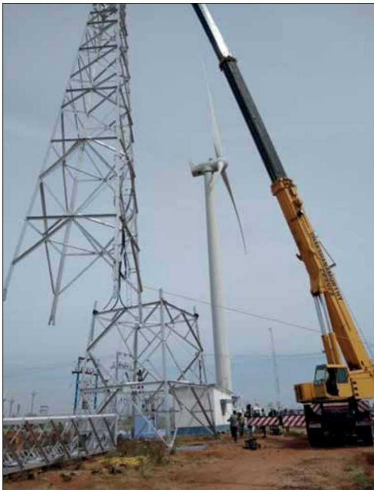
Fig. 10.13: DST Wind Turbine Instrumentation Work at Kayathar Research Station
