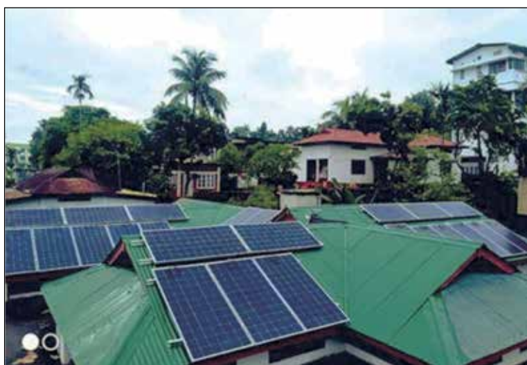
Fig. 8.1 : Solar Rooftop Installations at IIT, Guwahati
