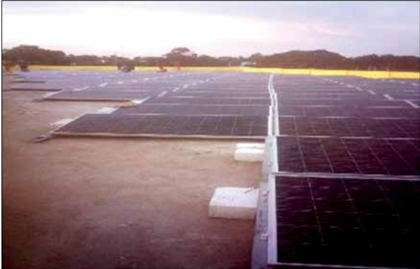
Fig. 3.7: Off-Grid Solar Power Plant for Temple Illumination
