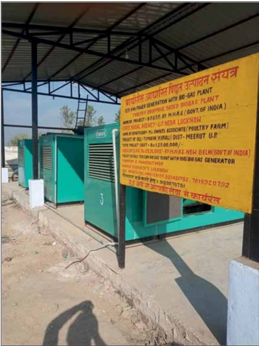
Fig. 5.1 Poultry dropping based Biogas plant
