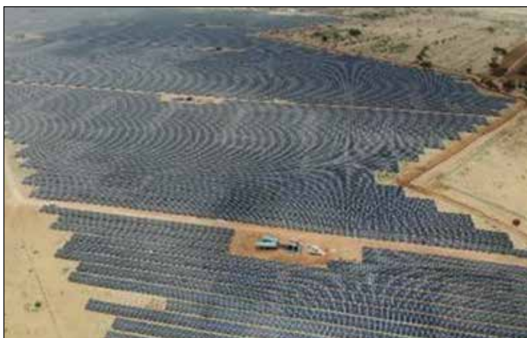
Fig. 10.22: 300 MW Solar Projects installed under ISTS IV tender in Karada, Jaisalmer
