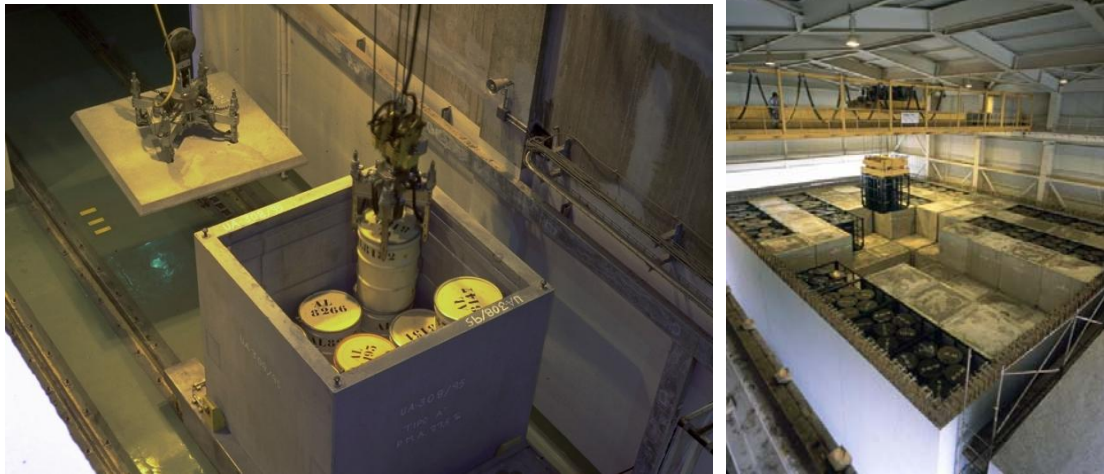
Figure 5. a) Loading radioactive waste packages of LLW and ILW into disposal containers. b) Loading disposal containers into the storage vaults.
