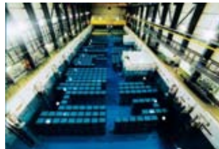
Irradiated Fuel Storage at La Hague Plant.
