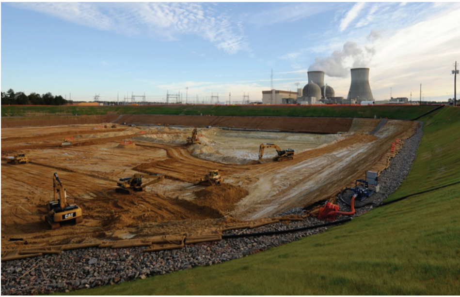
Site preparation already has begun for Vogtle 3 and 4, as shown above. Fortunately, investing in renewable energy and energy efficiency would eliminate the need for this high-cost, high-risk generation project.
