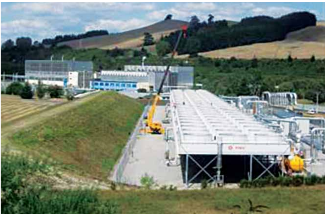
Figure A5.7: Bottoming 17-Megawatt Binary Plant (Foreground) at Wairakei, New Zealand
