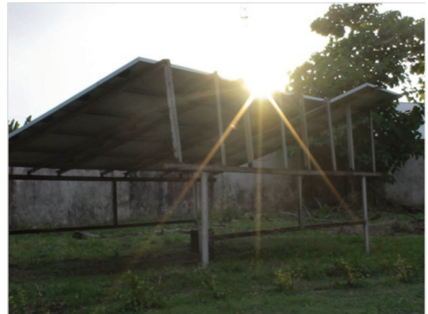
Figure 5.1: Solar water project, Delta State, incorrectly installed
