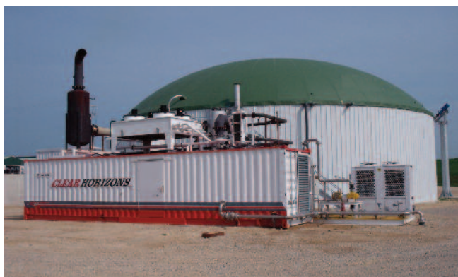
Figure 6. Complete-mix digester. (Courtesy of Leo Maney, Clear Horizons LLC).
