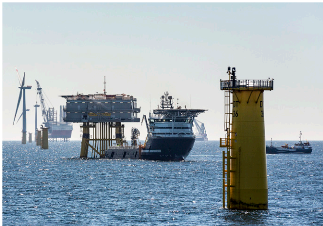
The offshore wind farm DanTysk while under construction in 2014. The 288 MW installation, owned by Vattenfall, is in the German North Sea.
