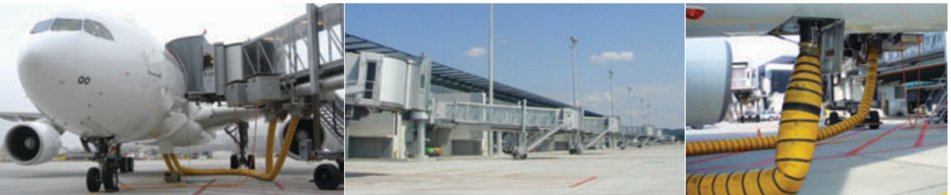
Fixed electrical ground power and air conditioning
