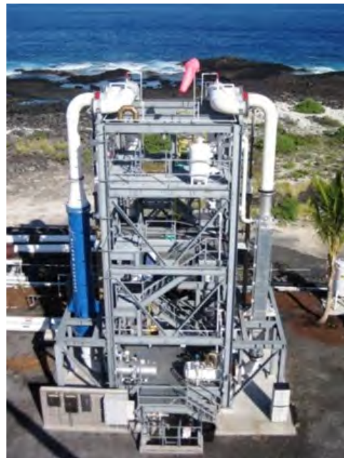
OTEC heat exchanger test facility at NELHA
