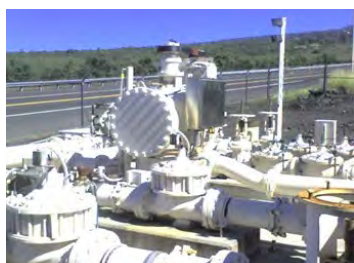
Hawaii County Dept. of Water Supply’s 45-kW in-line hydro plan in Kona
