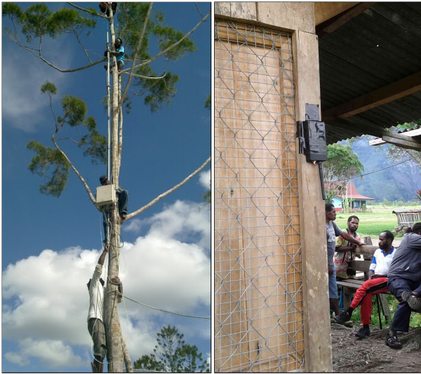
Figure 4: The installation locations of the BTS and a WUR.
