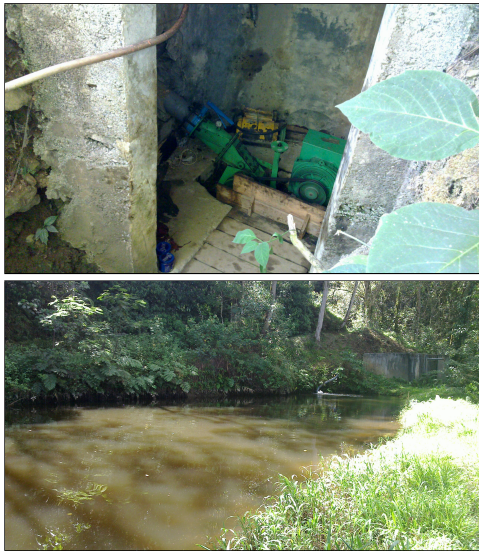
Figure 2: The hydroelectric generator and water reservoir.
