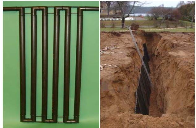
Fig. 8. Fence collector and its installation.
