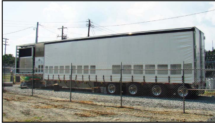
Figure 4-14 Premium Power’s 0.5-MW/2.8 MWh TransFlow 2000 Transportable Zinc-Bromine Energy Storage System, to be tested by EPRI and a utility consortium.
