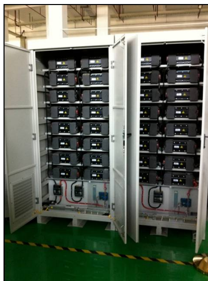
Figure 8 A 50-kWh BYD Li-ion Battery System Planned to be Tested at EPRI's Knoxville, Tenn. Smart Grid Laboratory in 2011.
