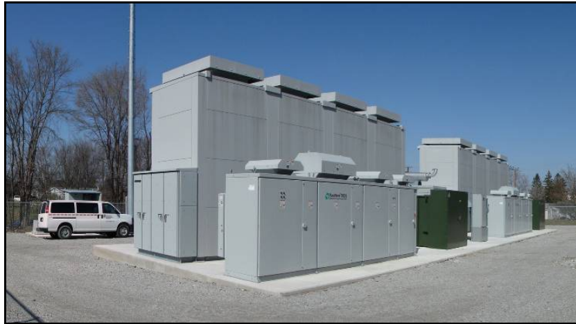
Figure 4-11 AEP Distribution Substation with Sodium-Sulfur Unit
