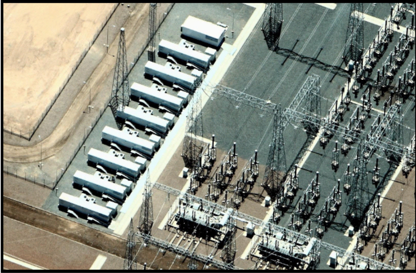
Figure 7 Commercial operation of a 12-MW frequency regulation and spinning reserve project at AES Gener's Los Andes substation in the Atacama Desert, Chile. The system uses A123 Systems' Li-ion Hybrid Ancillary Power Units (Hybrid-APUs™).
