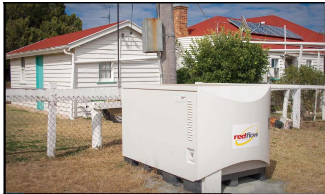
Figure 4-13 These 5-kW/20-kWh Community Energy Storage (CES) Systems by RedFlow Power and Ergon Energy of Australia will be linked by a Smart Grid network to provide megawatt-scale storage on the electricity grid.
