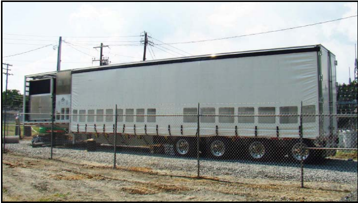
Figure 4 Premium Power's 0.5-MW/2.8 MWh TransFlow 2000 Transportable Zinc-Bromine Energy Storage System Preparing for Demonstration by EPRI.
