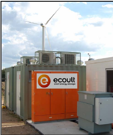
Figure 4-8 Phase 1 of Ecoult 1-MW/1-MWh UltraBattery system at Hampton Wind Smoothing Project in Australia (Source: Ecoult).
