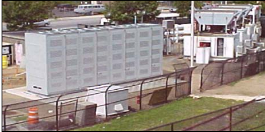
Figure 4-10 NYPA 1.2-MW/7.2-MWh Sodium-Sulfur Battery Facility
