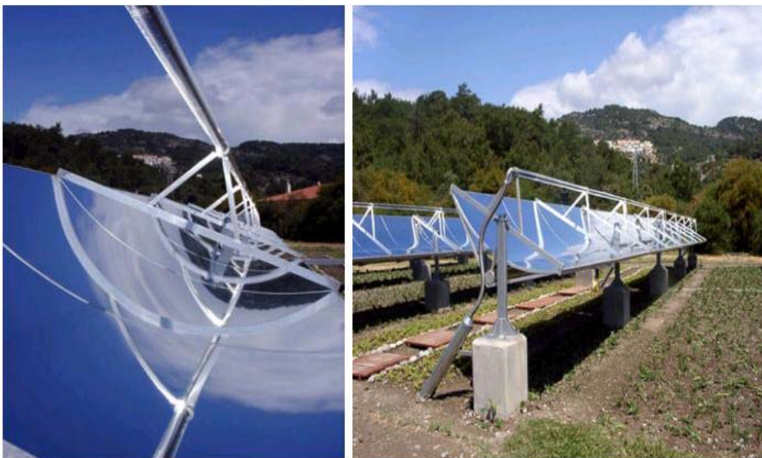
Figure A-42: Parabolic trough collector field for heating and cooling purposes of the Iberotel in Dalaman, Turkey. Source: /SOLITEM 2004/
